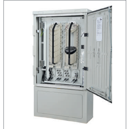
KVZ Street Cabinet with single fibre management
